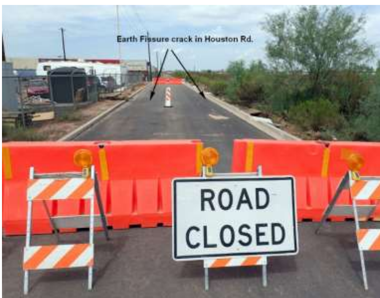
Figures 1a-b. W. Houston Road closed due to damage from earth fissure. Earth fissure nicely exposed adja- cent to W. Houston Rd. Photos by Joe Cook.
