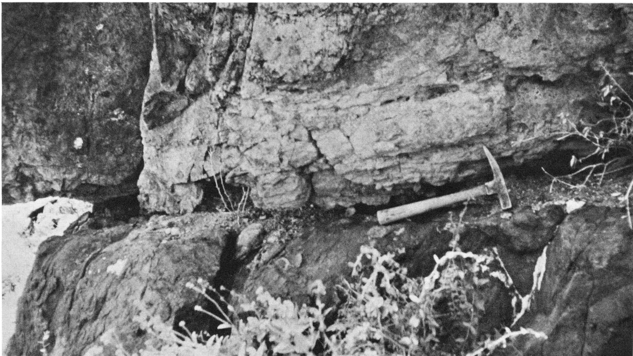
D. South end of Vulture Peak ridge (sec. 16, T. 6 N., R. 5 W.). View of west-dipping, low-angle, listric normal fault which places shattered, silicified, Tertiary rhyolite on intensely brecciated Precambrian(?) granite. Hammer rests on half-meter-thick ultrapotassic rhyolite dike intruding the fault plane.
