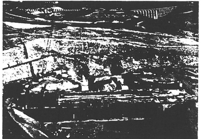
The Waddell Pumping-Generating Plant structure is eighty percent complete. The plant will pump Colorado River water through the two tunnels behind it for storage in Lake Pleasant. A small amount of hydroelectric energy will be generated when the water is released back to the CAP.
