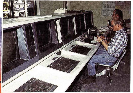
Flash Furnace Controls
