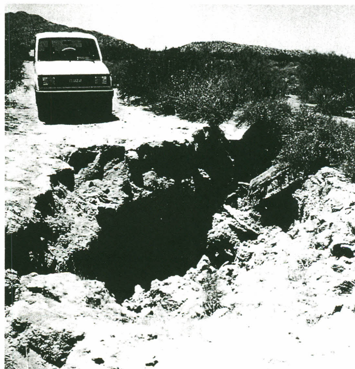
Figure 4. An earth fissure cut this road in Pinal County several miles east of Chandler Heights. Photograph by R. C. Harris.
